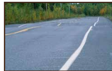
Frost heaves on the Richardson Highway.
