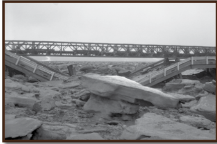
Earthquake damage to the Seward Highway bridge over Twentymile River near Portage on Turnagain Arm, following the earthquake of March 27, 1964.
