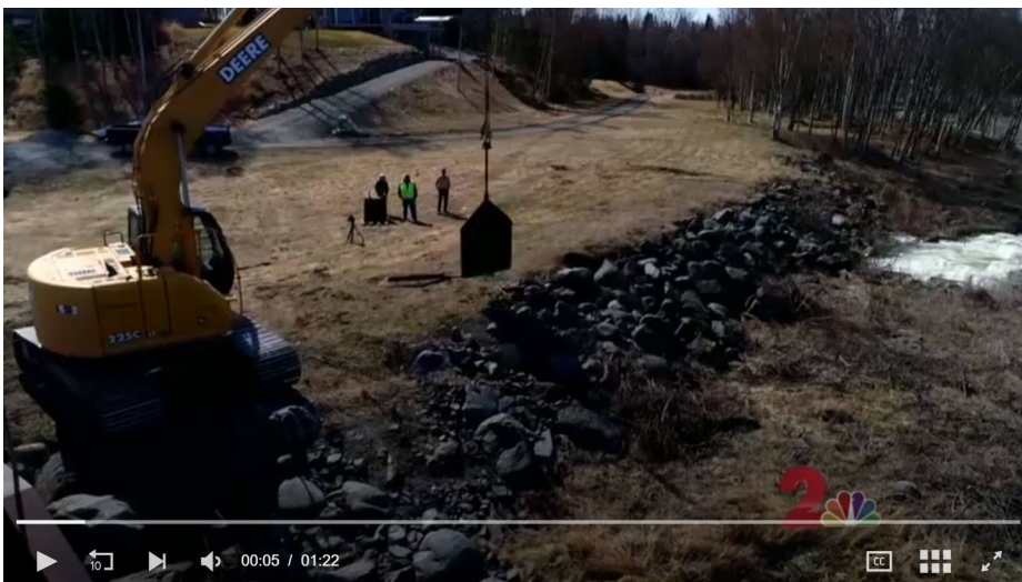
Screenshot of KTUU news segment showing AWWU-operated machinery lifting gates to the Campbell Lake dam.
