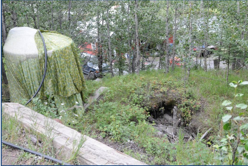
Figure 12: Photograph by Kevin Sorensen, DNR PAAD Unit, August 12, 2010. Photo taken from the off the roadway. To the left is the water tank. The red building in the background is the Mess Hall and the hole is the collapsed roof of the cache filled with debris.
