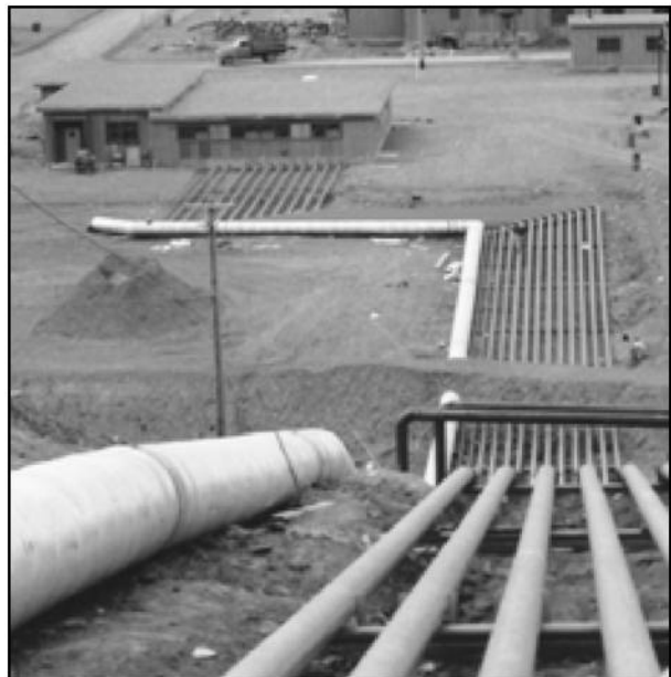
Figure 26. Pipes leading from manifold building to tank farm. Tok Terminal. NARA.
