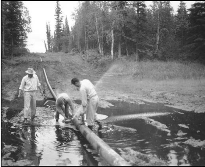
Figure 14. Pipeline break located near MP 498.8. Break was discovered during test period and was repaired. NARA.
