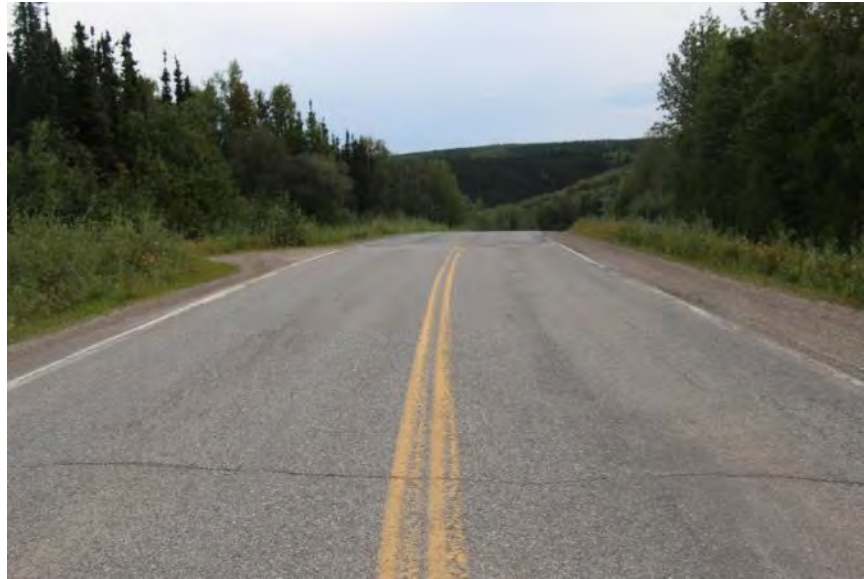
Figure 3. Typical roadbed in hilly terrain. View facing northeast.
