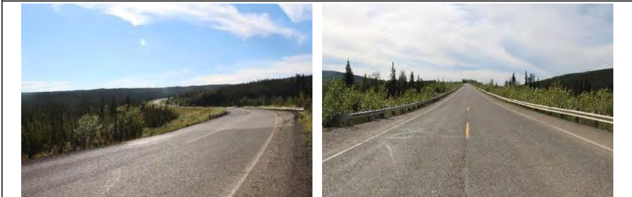
Figures 12 (view facing east) and 13 (view facing north). Typical roadbed showing extent of elevated embankment due to borrow/fill.
