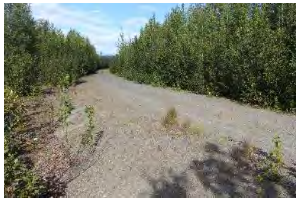
Figure 52. Roadbed and embankment reflective of pre-1959 period of significance. View facing north.
