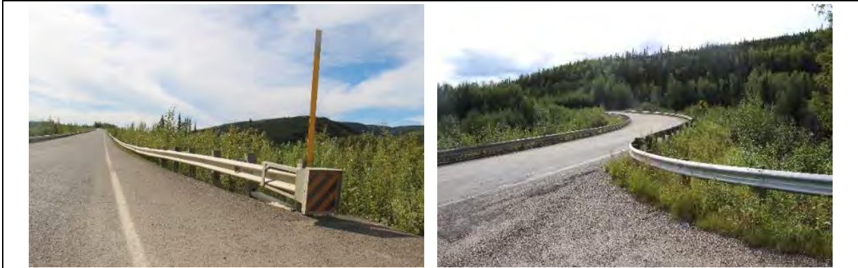
Figures 14 (view facing northeast) and 15 (view facing east). Examples of replacement guard railing.
