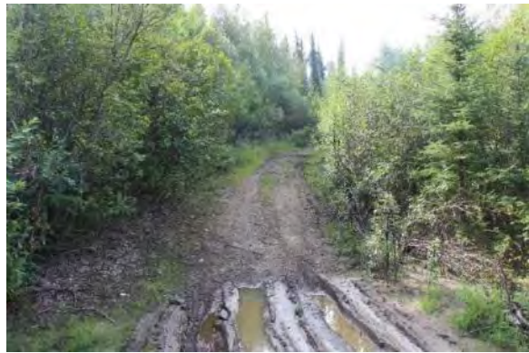
Figure 28. Example loss of embankment (unmaintained). View facing east.
