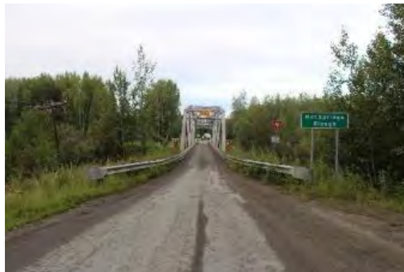
Figures 39 (view facing south), 40 (view facing north), and 41 (view facing south). Paved roadbed and 1961 overhead truss bridge in Manley Hot Springs.
