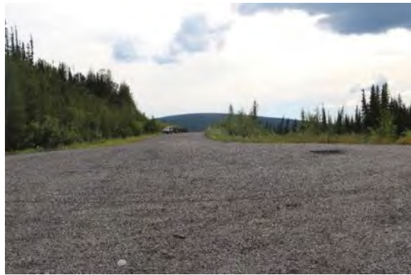
Figure 26. Example loss of embankment and travel lanes (widening). View facing northeast.
