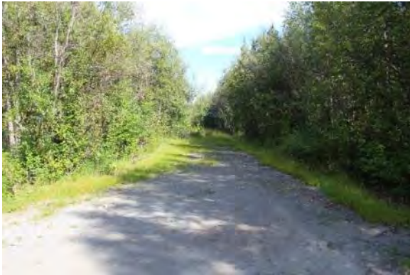
Figure 31. Example loss of embankment – north of the Tatalina River. View facing north.
