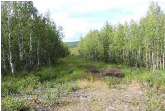
Figure 25. Example loss of embankment and travel lanes (obliteration of roadbed). View facing north.
