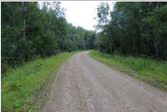
Figure 23. Southern portion of roadbed showing one travel lane and embankment reflective of pre-1959 period of significance. View facing north.
