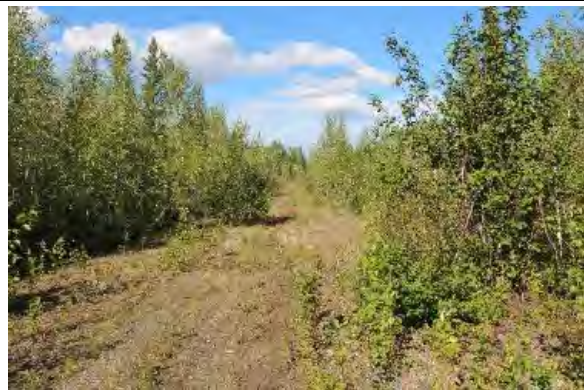
Figure 54. Example loss of embankment and travel lanes (obliteration of roadbed). View facing northwest.
