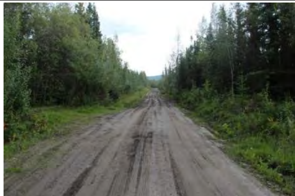
Figure 24. Northern portion of roadbed showing two travel lanes and embankment reflective of pre-1959 period of significance. View facing southeast.
