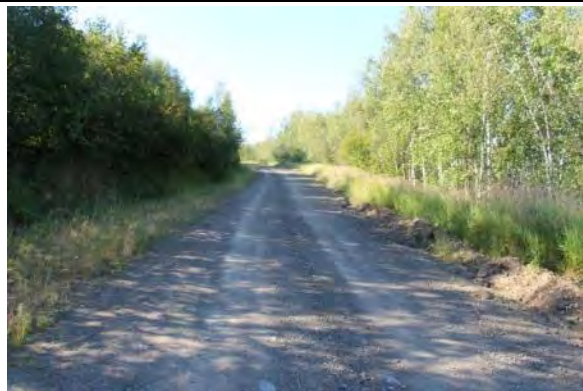
Figure 34. Gravel roadbed, one travel lane, and embankment reflective of pre-1959 period of significance. View facing southwest.
