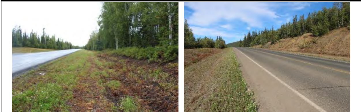
Figures 10 (view facing southeast) and 11 (view facing northeast). Typical roadbed showing extent of wide embankment.
