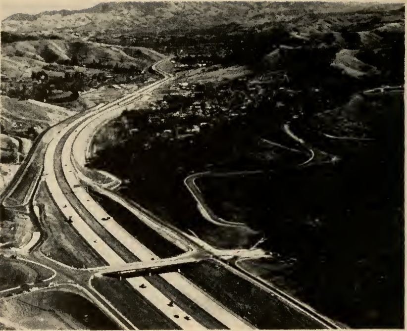
This 2-mile section of 6-lane freeway in California was completed during the year with Federal-aid "D" funds, replacing a congested 4-lane road built in 1943. The route connects Oakland with rapidly developing areas to the east, and is already carrying 40,000 vehicles daily.
