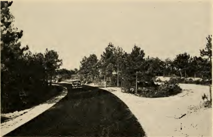
This 4-mile Federal-aid secondary project in South Carolina was built in Aiken County at a cost of $12,250 per mile, using local sand-clay soil to advantage as a base course for the 20-foot bituminous surface. A bad curve in the old road, eliminated by the improvement, appears at the right. Road-user savings in the next 15 years were estimated at $43,000.
