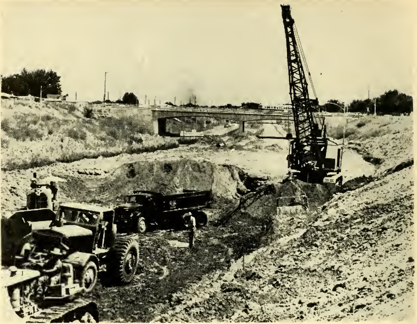
The last gap in the Valley Highway, the Interstate route through Denver, Colo., was under construction.
