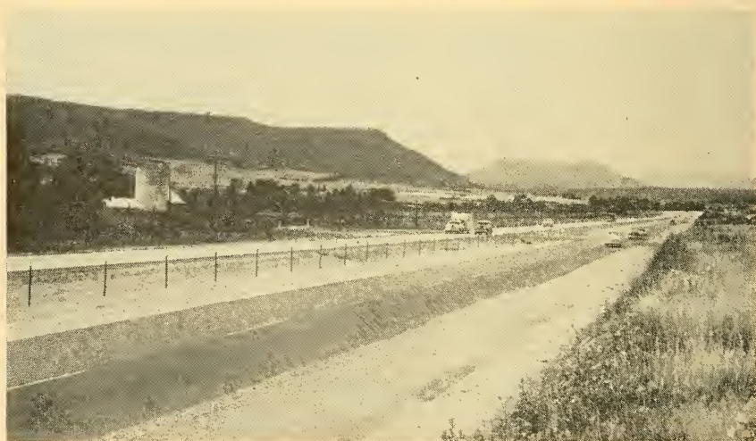
U. S. 85 and 87 between Denver and Pueblo, Colo., is being converted to a four-lane highway by construction of a new road parallel to the old road. The latter is being improved wherever necessary.
