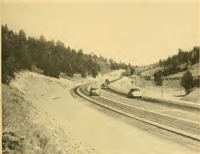
A newly built part of the interstate system over Sherman Hill in Wyoming, highest summit on U. S. 30
