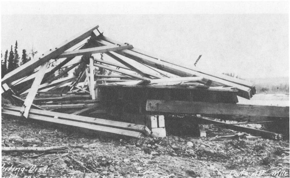
Bridge, with 100-foot span over the Gulkana River, at mile 128, Richardson Highway, was carried away by ice, May 9, 1933. Ray Huddleston Collection, UAF.
