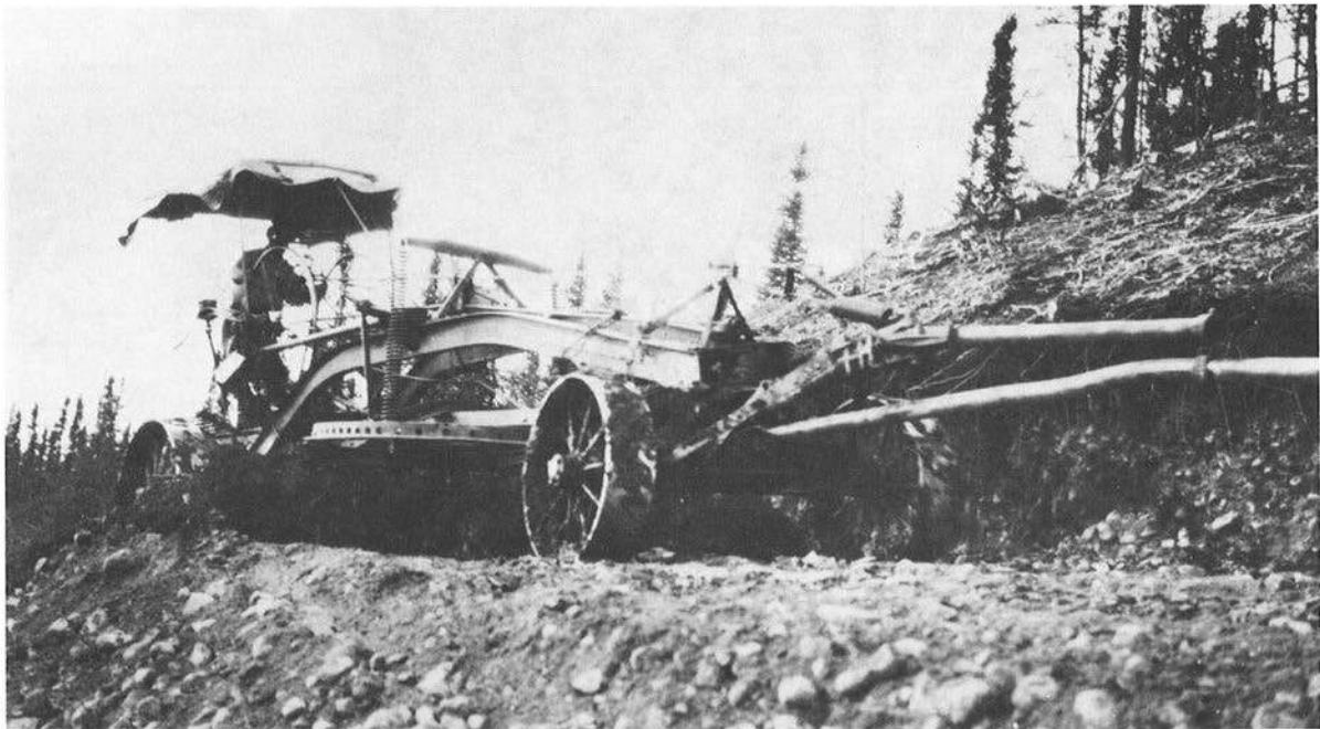
Twelve-foot grader at work on the Gulkana-Chisana Road, mile 49, 1931. Ray Huddleston Collection, UAF.
