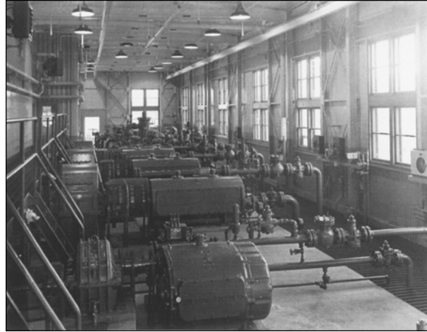
Figure 22. Mainline pumps. Tok Terminal. Courtesy George Lyle.
