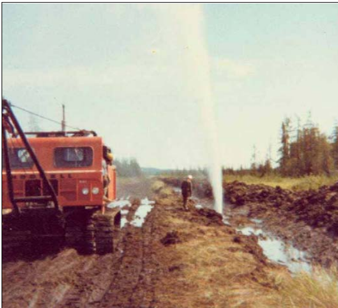
Figure 40. Water shooting out of a bullet hole during pipeline repairs.
