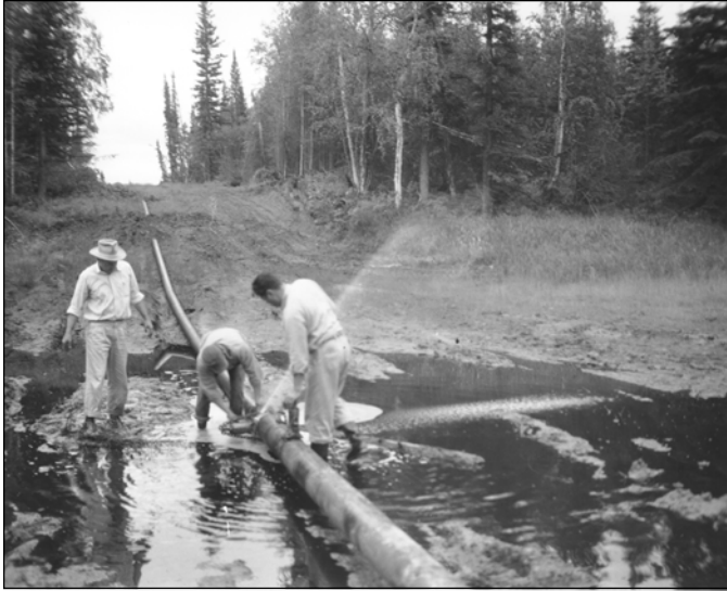
Figure 14. Pipeline break located near MP 498.8. Break was discovered during test period and was repaired. NARA.
