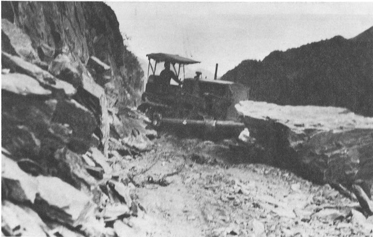
Bulldozer moving rock slide, mile 43½ on the Richardson Highway, Valdez district, August 1940. Ray Huddleston Collection, UAF.
