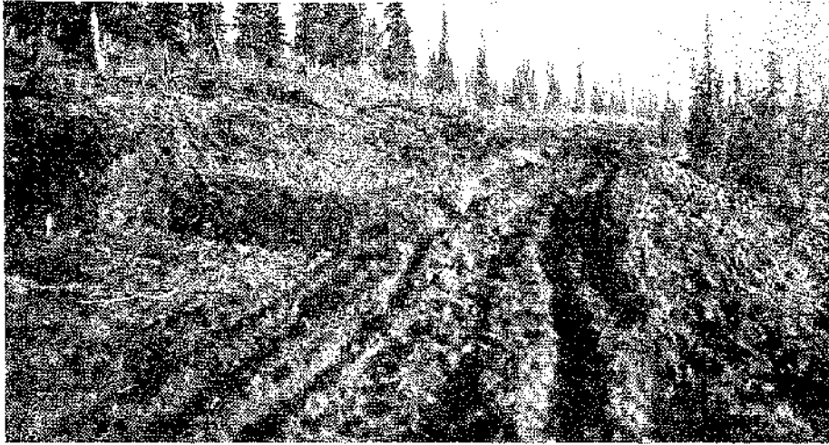
THAWING OF SUBGRADE AFTER STRIPPING---SOUTHWESTERN DISTRICT
