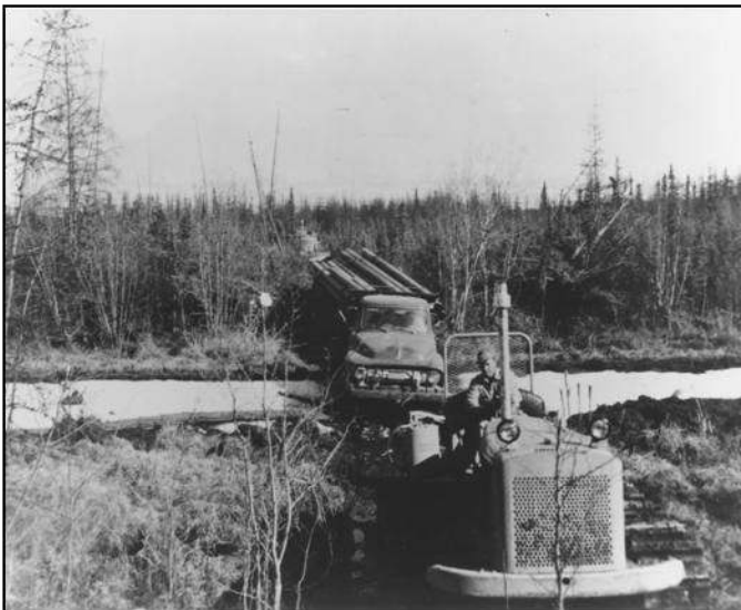
Figure 4. Push and Pull assistance was necessary to bring piping to the places needed in tundra swamp crossing. NARA.
