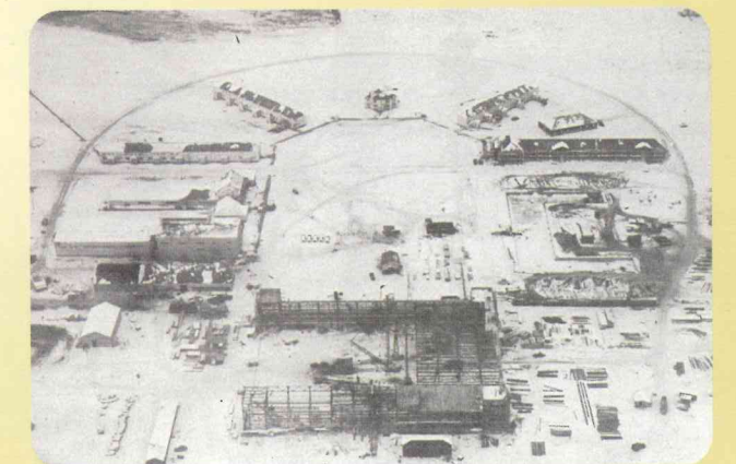
An aerial view of the Headquarters area in 1940. Hangar One is under construction in the foreground, while the foundation was being laid for the Air Corps Barracks and the BOQ was receiving finishing touches. AAF photo.
